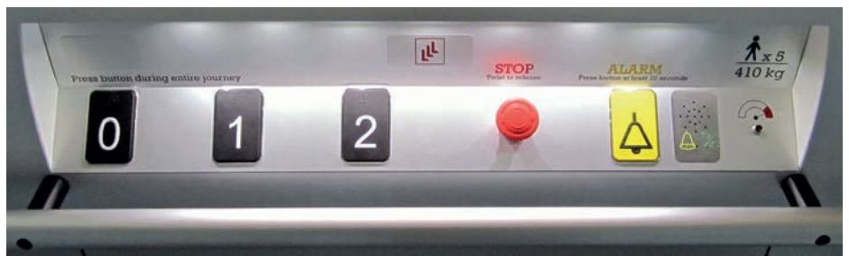
Superior 3 Flexi Platform & Goods Lift control panel
