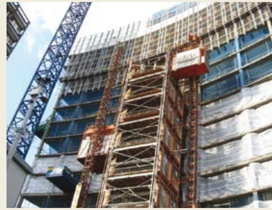
An aluminium tower supports the three hoists on the Strata Tower job site in London.
