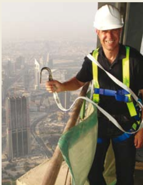
Pega project manager Pavel Policar, pictured at 625 m, on site to place the last, permanent hoist in November.
